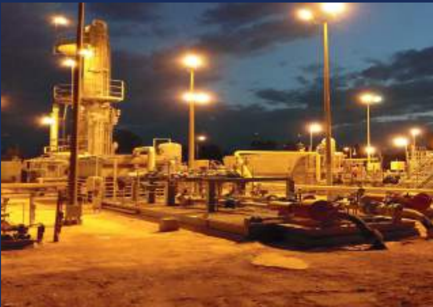
Kingdom of Saudi Arabia, Government Qurayyah combined cycle power plant
