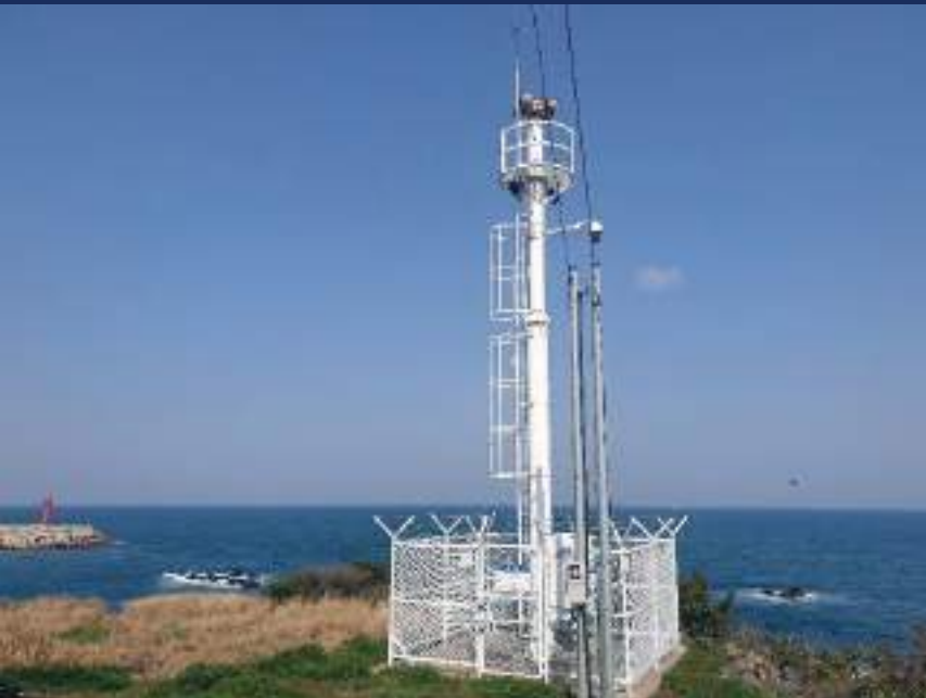
Greece, MOD Coastal security system
